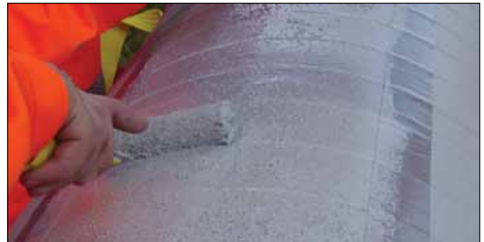
4. Apply anti-slip walkway surface to the topside of the wrapped main cables.
