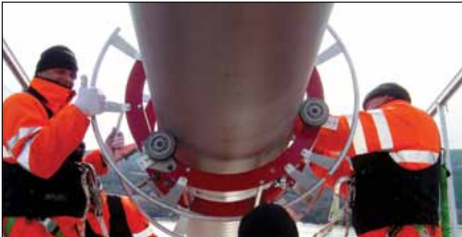
1. Use the Skewmaster™ wrapping machine to apply Cableguard™ between cable bands with a 50% overlap.
