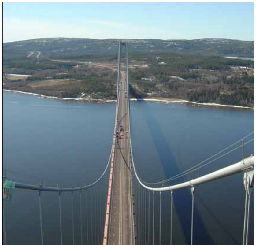
The Högakusten Bridge in Sweden was wrapped in 2005 and employs main cable dehumidification.
