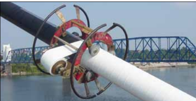
1. Use the Skewmaster™ wrapping machine to apply the Cableguard™ continuously with a 50% overlap.
